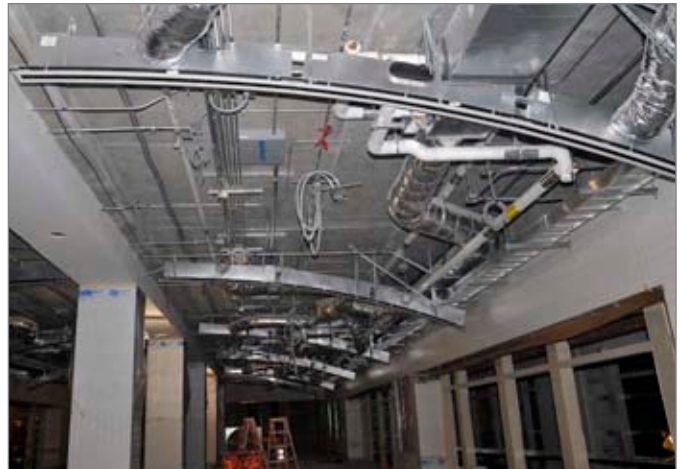
Installed curved DesignFlo.
