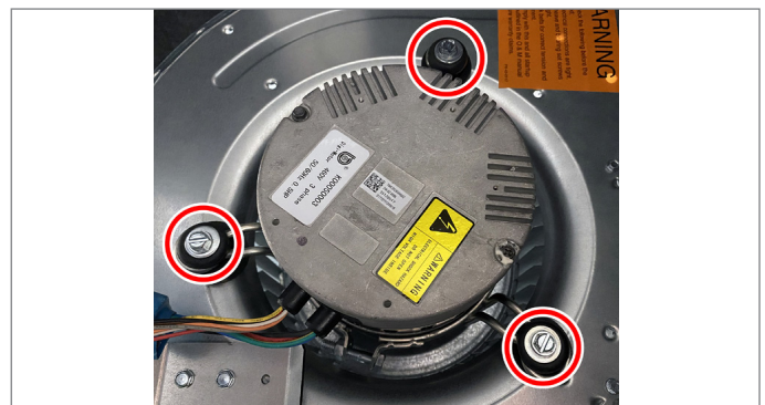
Figure 5d: Motor Access
